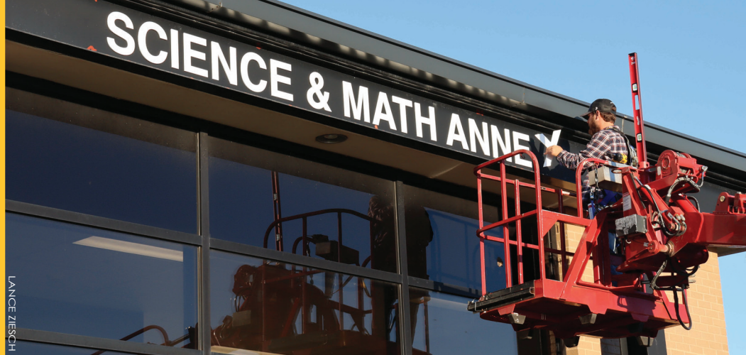
A worker from Miracle Signs installs new lettering on the east end of the Science & Math Annex on Sept. 27.
